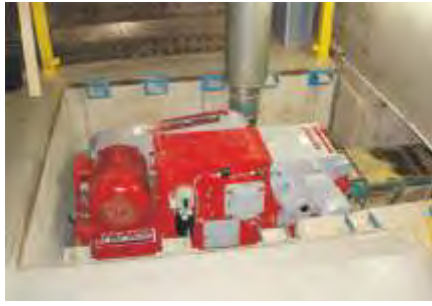
RHZ 400 S set up below ground
